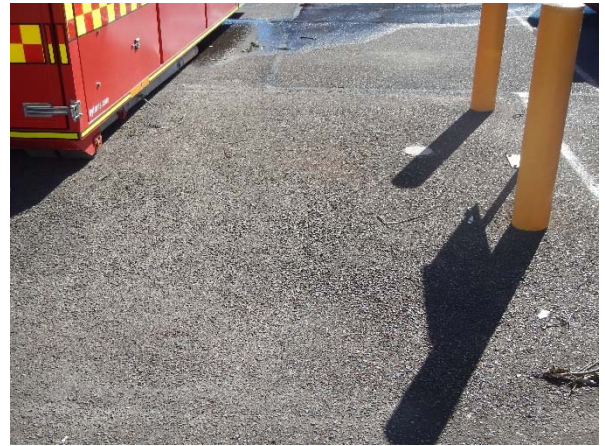
▲ Photograph 8: The possible area where the underground water storage tank is. Former points have been concreted in. Located in the southern area of the site near the fire training ground.
