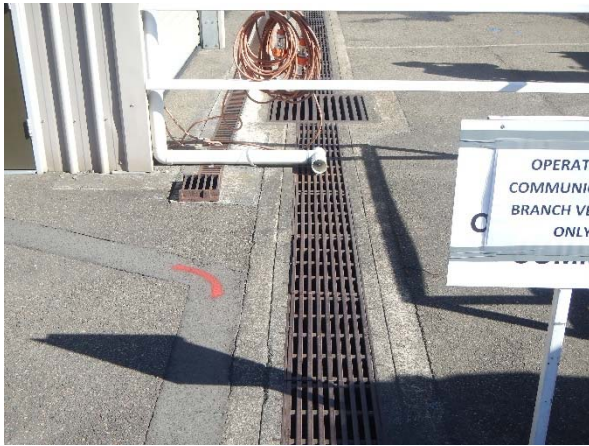
▲ Photograph 7: The drain the surrounds the fire training area that flows to an underground holding tank..
