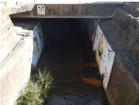
▲ Photograph 11: Facing north west of Sheas Creek culvert where the culvert runs underneath the site.
