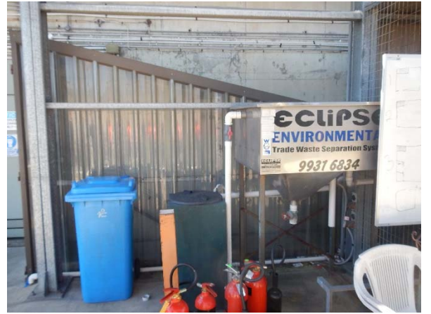
▲ Photograph 2: An interceptor for the site, located in the former truck wash area.
