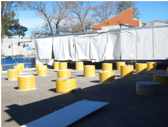
▲ Photograph 9: Facing west in the southern area of the site - construction in progress.
